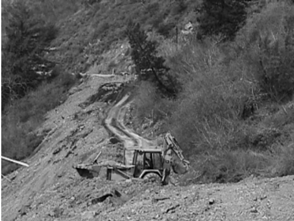
Mudslide at Grandpa's Elbow, 1998 (Photograph courtesy James Kimball, www.surcoast.com )
