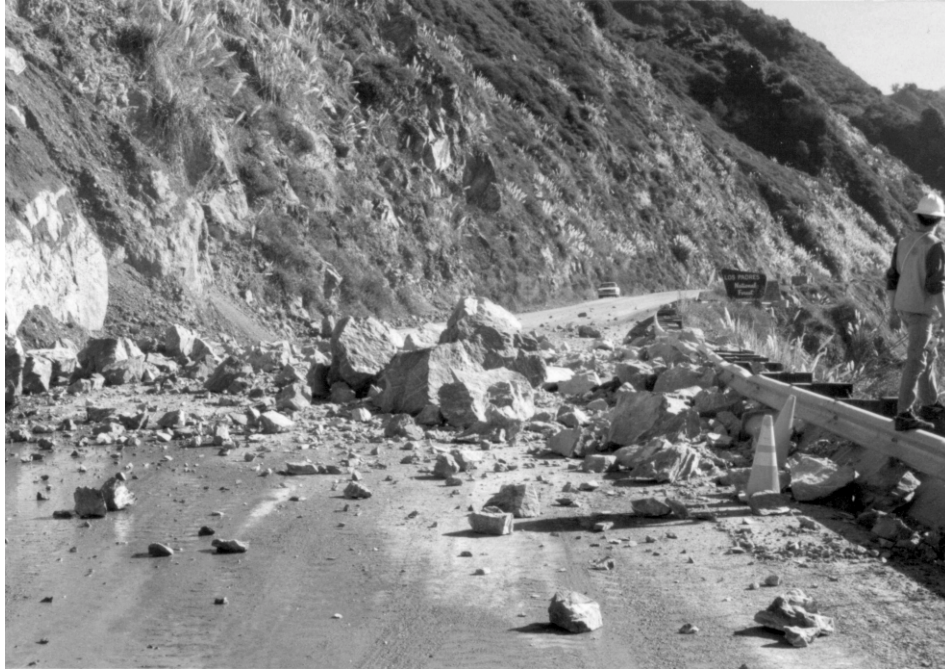
Rockslide at “Big Slide,” December 15, 1996 ( Photograph from Caltrans District 5 Maintenance Records )
