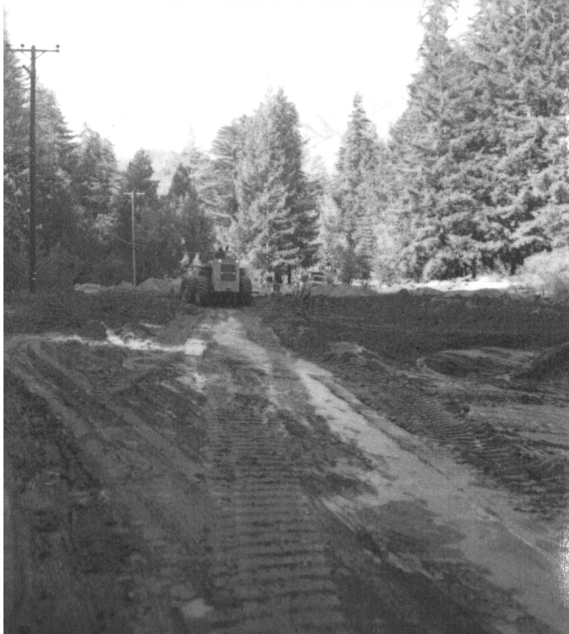
The Molera Slide, Big Sur Village, November 1972 (Photograph by Pat Hathaway, Pat Hathaway Photograph Collection, Monterey)
